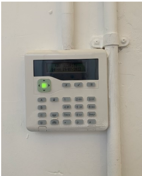
Alarm system next to front door
